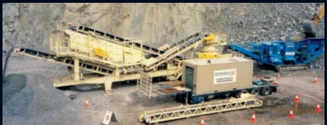
Mobile Crushing Plant and Secondary Circuit
