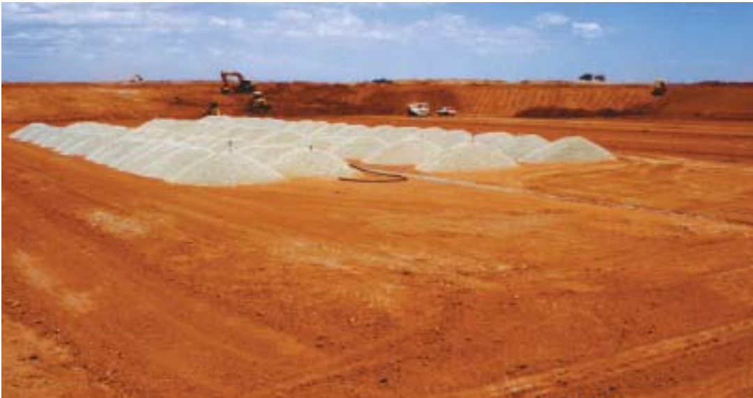
Recycled Concrete Aggregate baled and ready to be laid out in the first cell at Dublin
